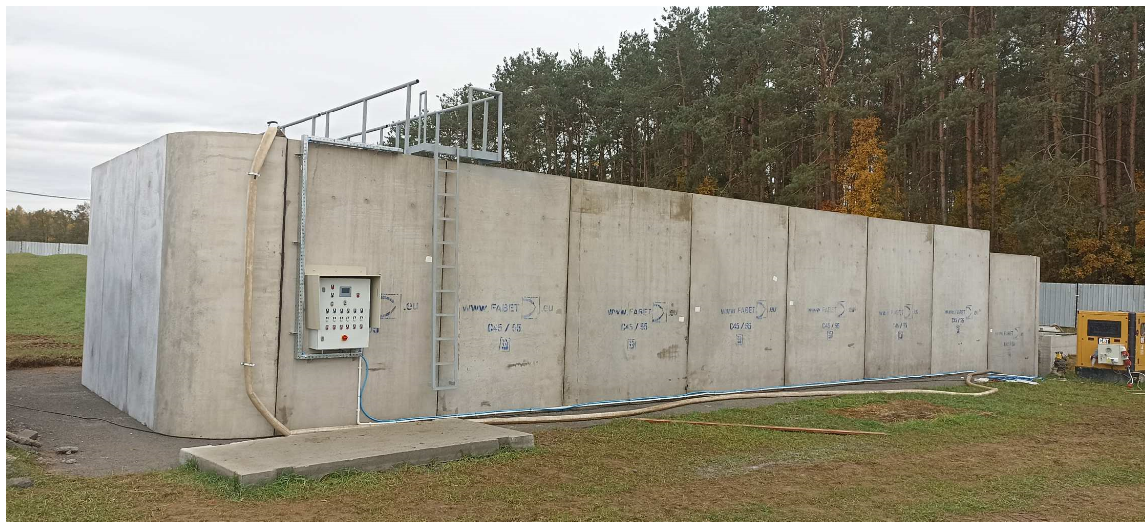
Figure 1: Physical model of the retention tank with installed sluice gates and control panel
